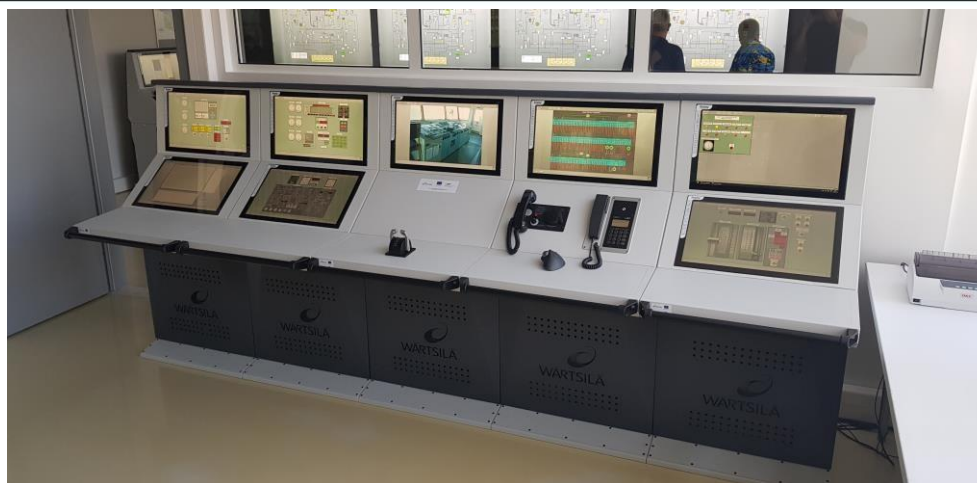
Figure 8. Simulator of the control desk in the engine control room
