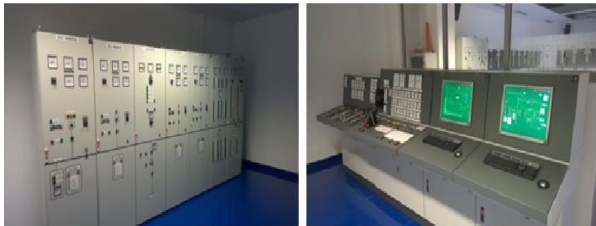
Figure 13. ER control room of the ECR KONSBERG simulator
