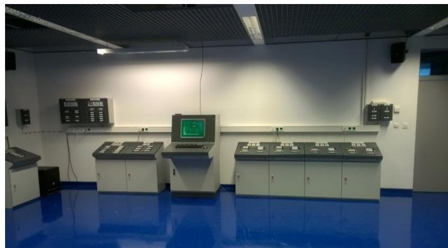
Figure 14. Control desk of the engine room
