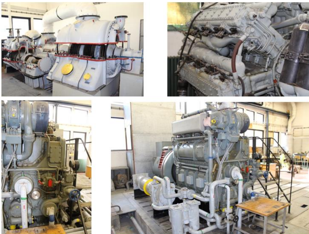
ENGINE ROOM CABINET (Lora)
