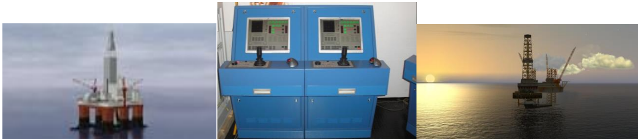
The location of the DP consoles on the bridge
